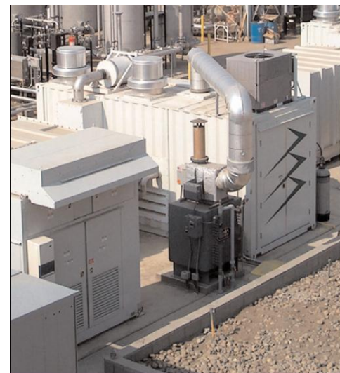
Photo from FuelCell Energy, Spotlight on the City of Tulare, CA fuel cell at a wastewater treatment plant.
