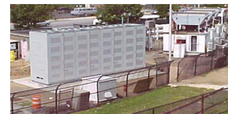
NYPA 1.2-MW/7.2-MWh Sodium-Sulfur Battery Facility
