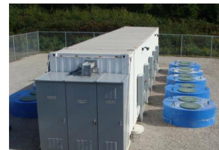
1-MW/15-min Beacon Power flywheel in an ISO ancillary service application
