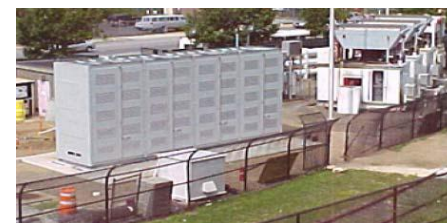
NYPA 1.2-MW/7.2-MWh Sodium-Sulfur Battery Facility
