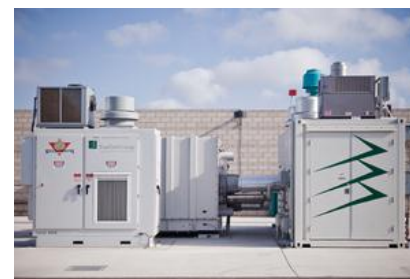
Fuel Cell Energy equipment at Gills Onions, Oxnard, California. Source: Biomass Power and Thermal Magazine
