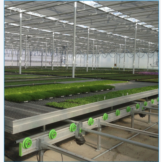
A thermal canopy attached to the greenhouse rafters descends at night, acting as insulation for Edible Garden's herb plantings, maintaining temperatures at the plant level.
